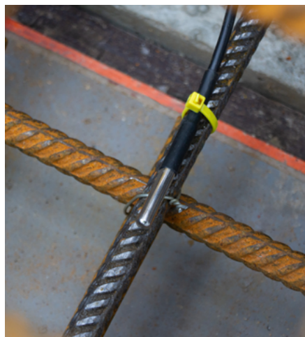
Figure 2: Digital Thermocouple mounted
